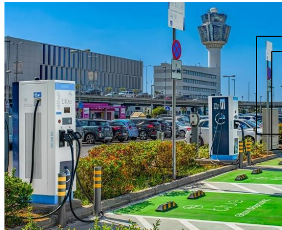
EV charging station
